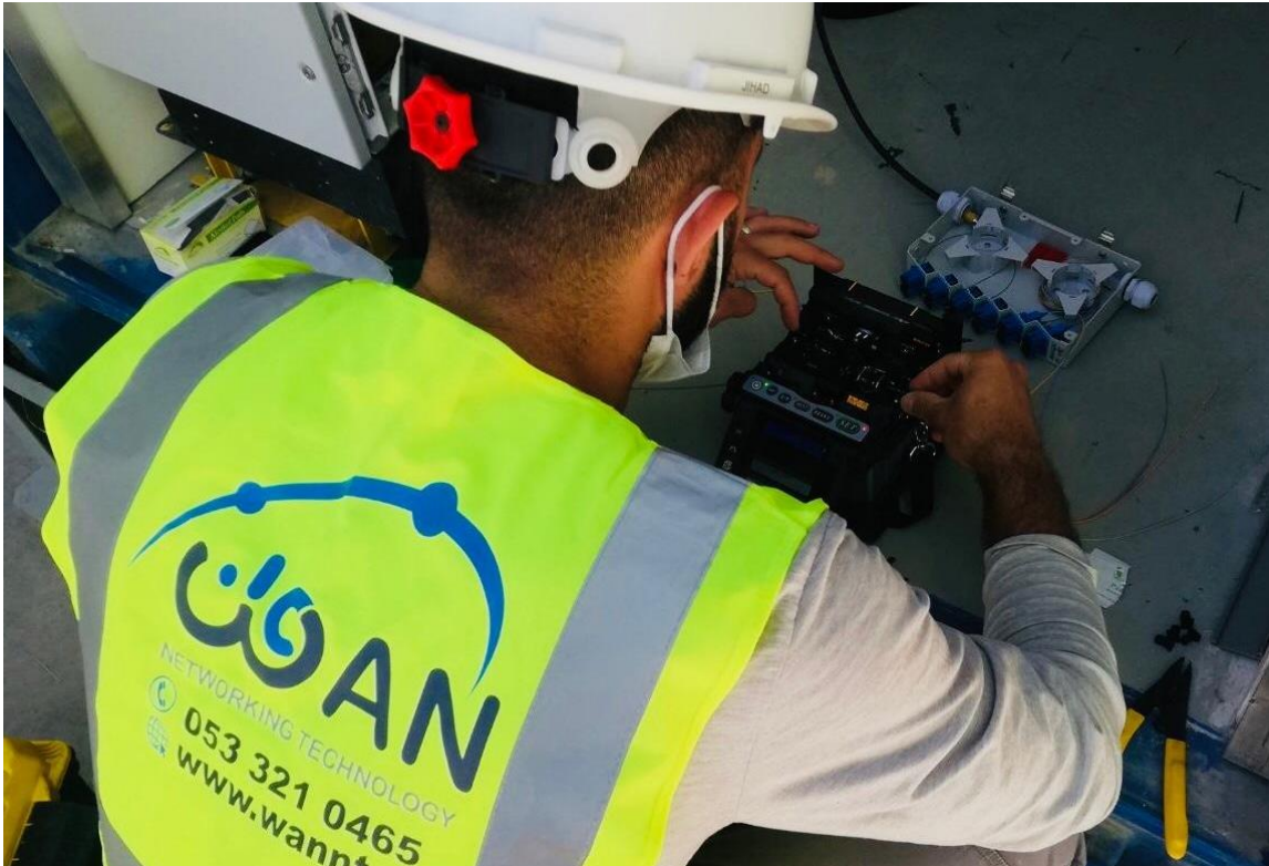
Fig. 3 Fiber Splice Process
